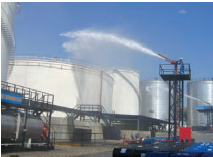
Firefighting Equipments in Marmara Terminal
