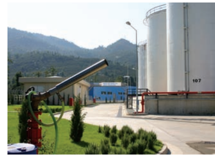
Firefighting Equipments in Giresun Terminal
